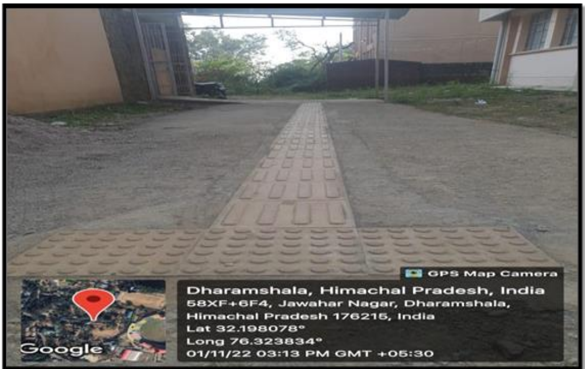
Photograph showing the facility of tactile path to create Divyangjan friendly environment at Central University of Himachal Pradesh
